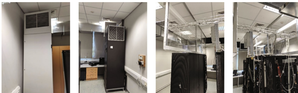
FIGURE 2 Energy Efficiency Upgrade of data center room (equipment and positioning).
