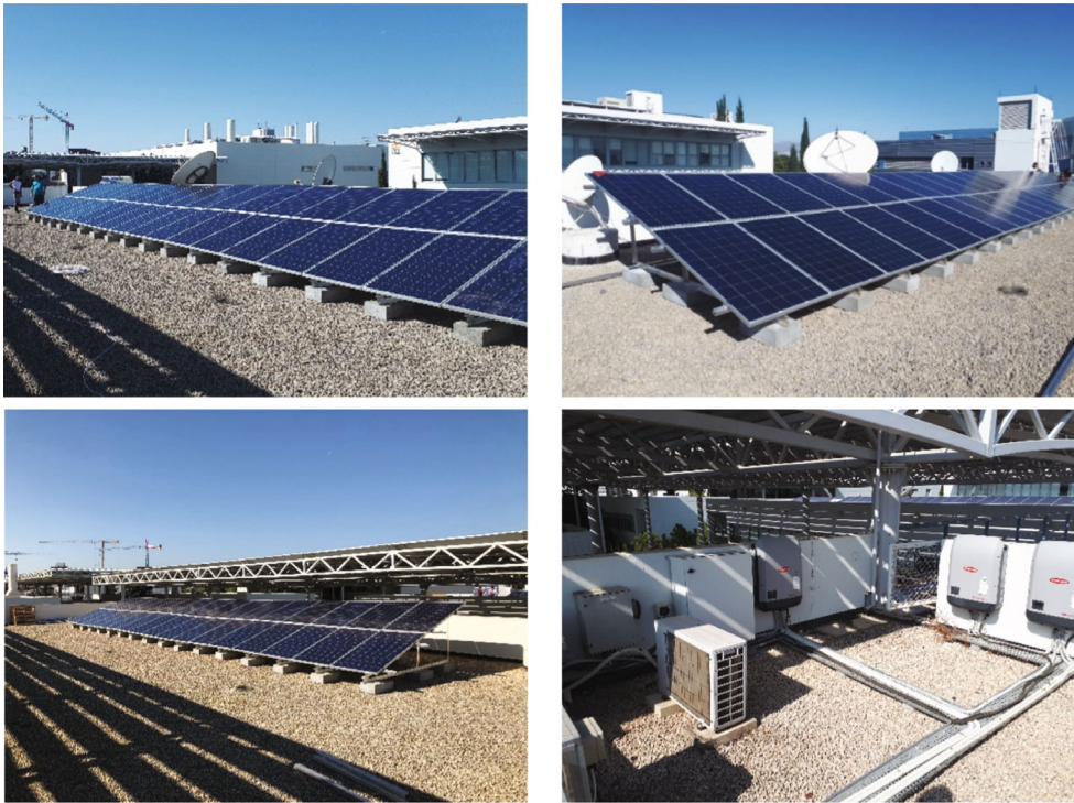
FIGURE 4 Outdoor photovoltaic installation.
